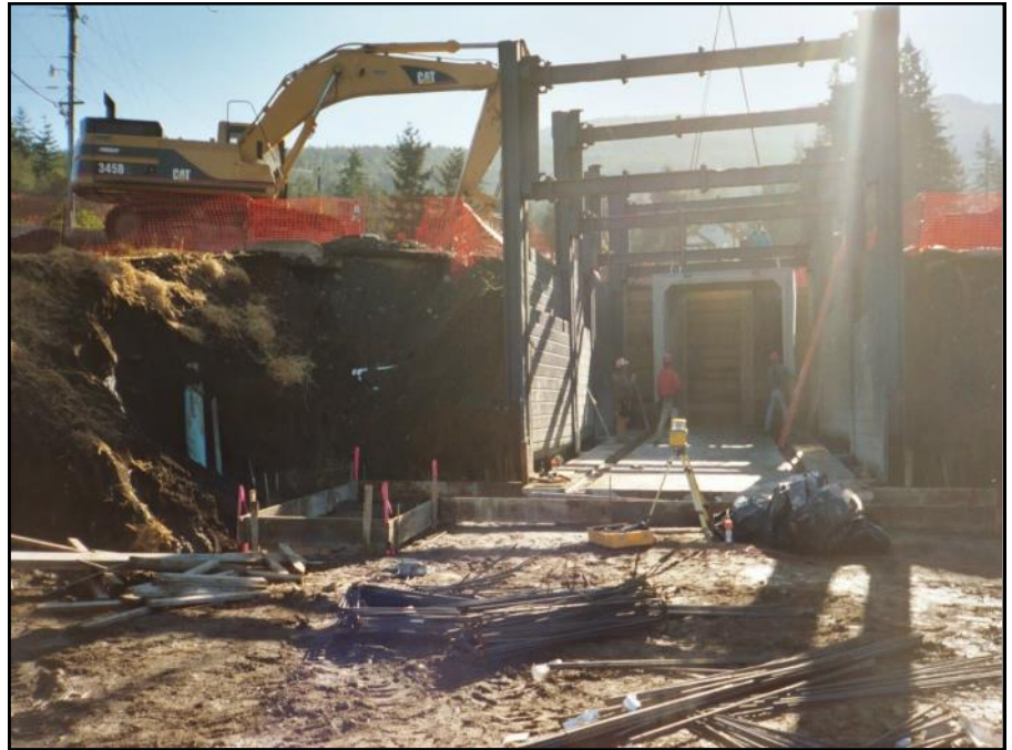
The Pedestrian-Service Cart Tunnel was completed 2004, and is used by staff and Tribal citizens who need to get safely across Highway 101.
