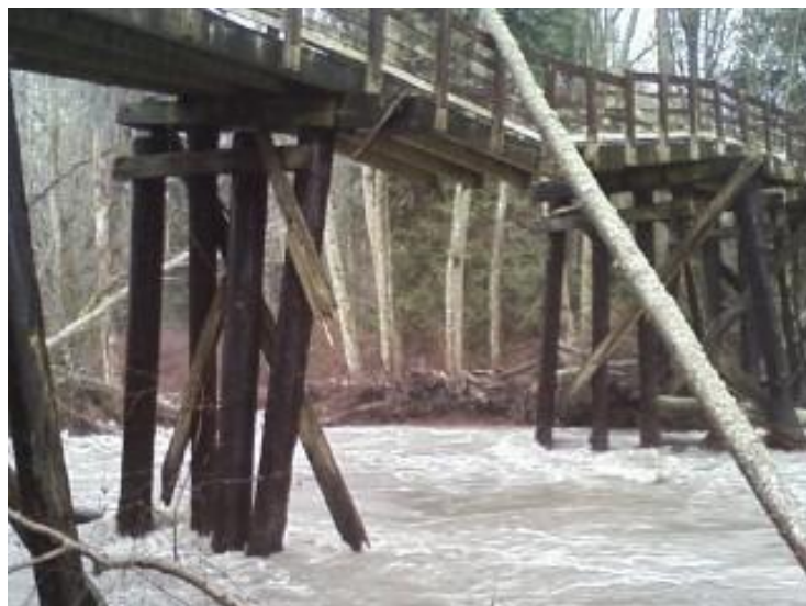
High water unearthed and snapped six pilings that held up the walkway over the Dungeness River .
