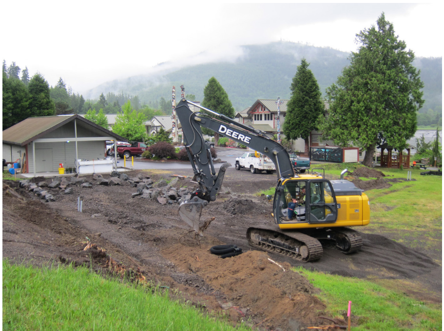
Jamestown Excavating staff reshaping the entrance to the Westrem property, where additional parking and the Veterans Memorial were built this year.
